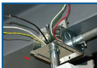
(2) Install cover plate on lighting fixture and slide it back into the box
